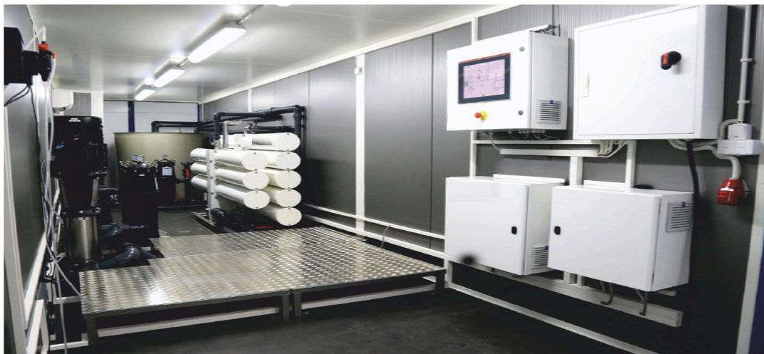
Brackish water RO plant 35m 3 /h
